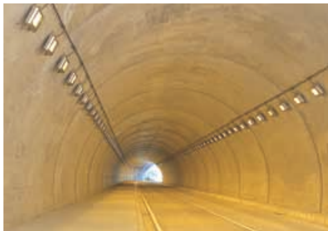
晴天時照明状況(全点灯) Lighting condition on fine days (All lights are on in full capacity)
