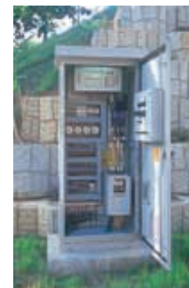
照明分電盤 Lighting panel
