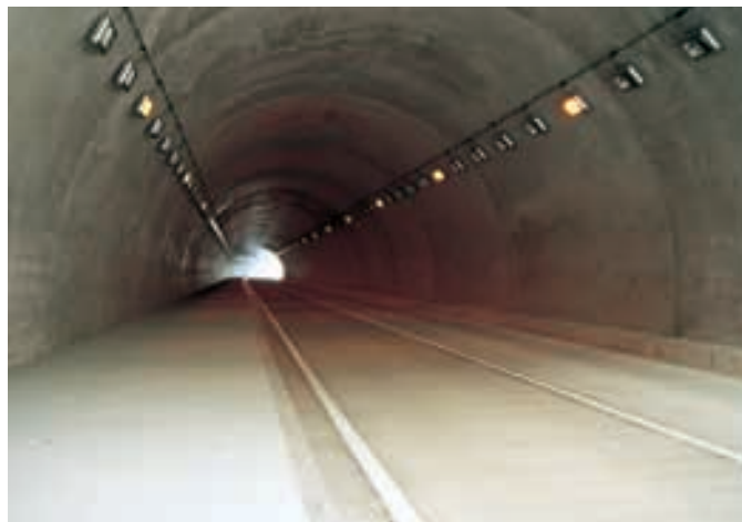
夜間時照明状況(基本照明のみ) Lighting condition at night (Basic lighting)
