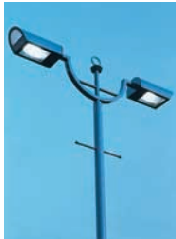
車道灯 A lamp on the roadway
