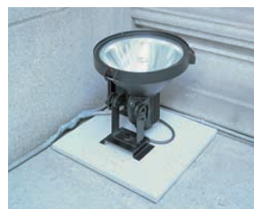
投光器アップ Closed-up photo of a floodlight
